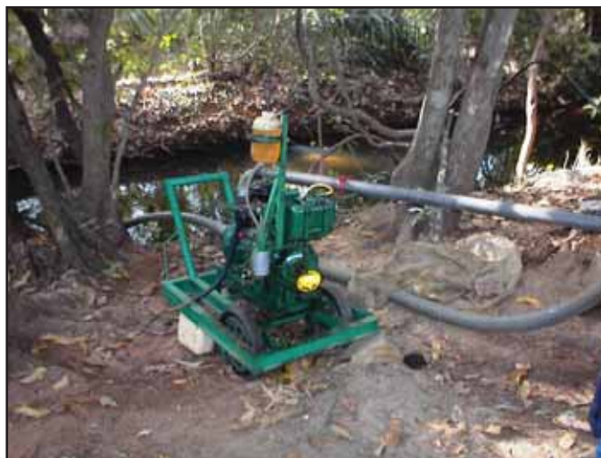
Figure 5 Small Mechanical Centrifugal Pump
