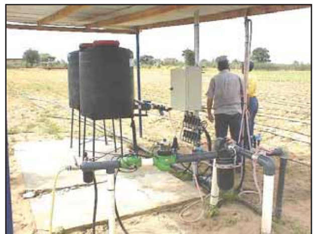
Figure 3 Drip Irrigation System
