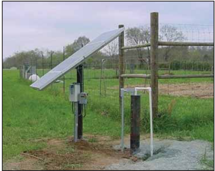
Figure 7 Solar-powered Electric Pump
